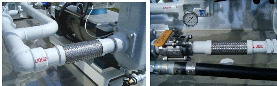
Fig. 8. Flexible Hoses used at Inlet and Outlet
